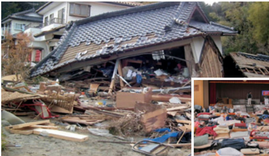
Collapsed house near the east coast of Honshu, Japan, following the earthquake and tsunami
