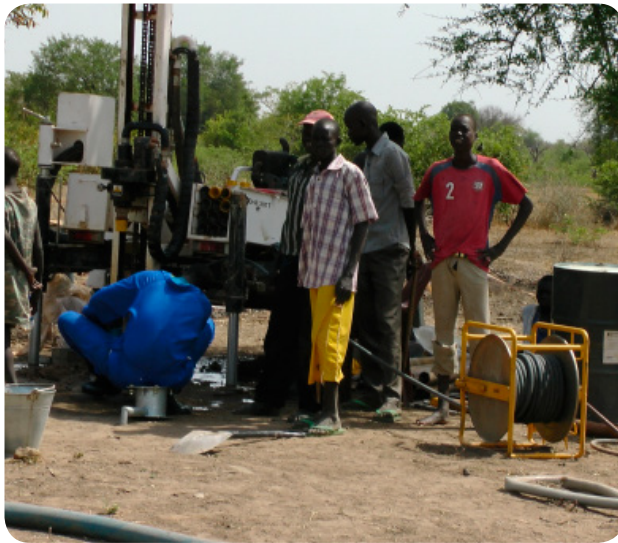
Contractors drill a borehole in Lurchuk village, Warrap state of South Sudan, as part of an earlier project by the Diocese of Wau.
